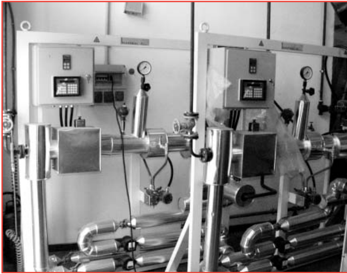
Steam control units supplying the preconditioner and the extruder.
